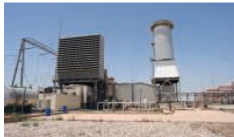
FIGURE 4. A example of a very large gas turbine installation. The air inlet filter and the exhaust gas stack are also shown.
