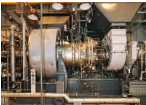
FIGURE 2. In an example of a modern gas turbine with good aerodynamics and advanced combustion technologies, this twin-shaft gas turbine achieves a useful power output of around 13–14 MW. Thus, this gas turbine model has been used for both power generation and mechanical drive. This is an example of a modern twin-shaft gas turbine that combines aero-derivative and heavy-duty technologies in one advanced gas turbine. The turbine permits an efficiency of about 35–36% for operation in a simple cycle. Adding a heat-recovery system will improve overall efficiency. This machine has an excellent power-to-weight ratio in its application range. (Photo used with permission from Siemens)
